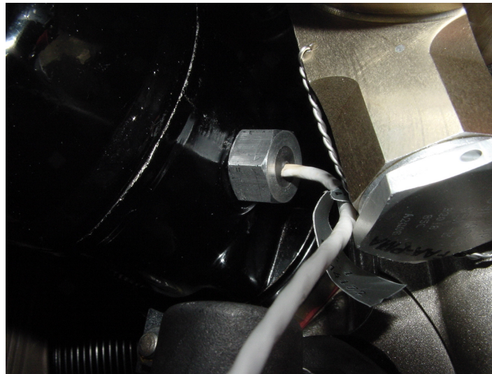
Figure 14-16 Magneto Tach Sensor Installed
